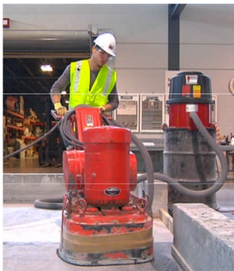
Worker milling granite floor indoors with milling machine and vacuum dust collection system (background). Photo courtesy of OSHA
